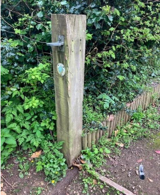
Photo 13. HU 10.1 (April 2025) Rotten Post
